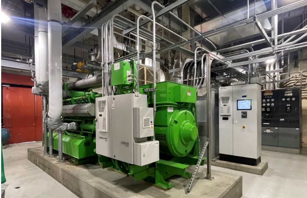
New cogeneration engine
